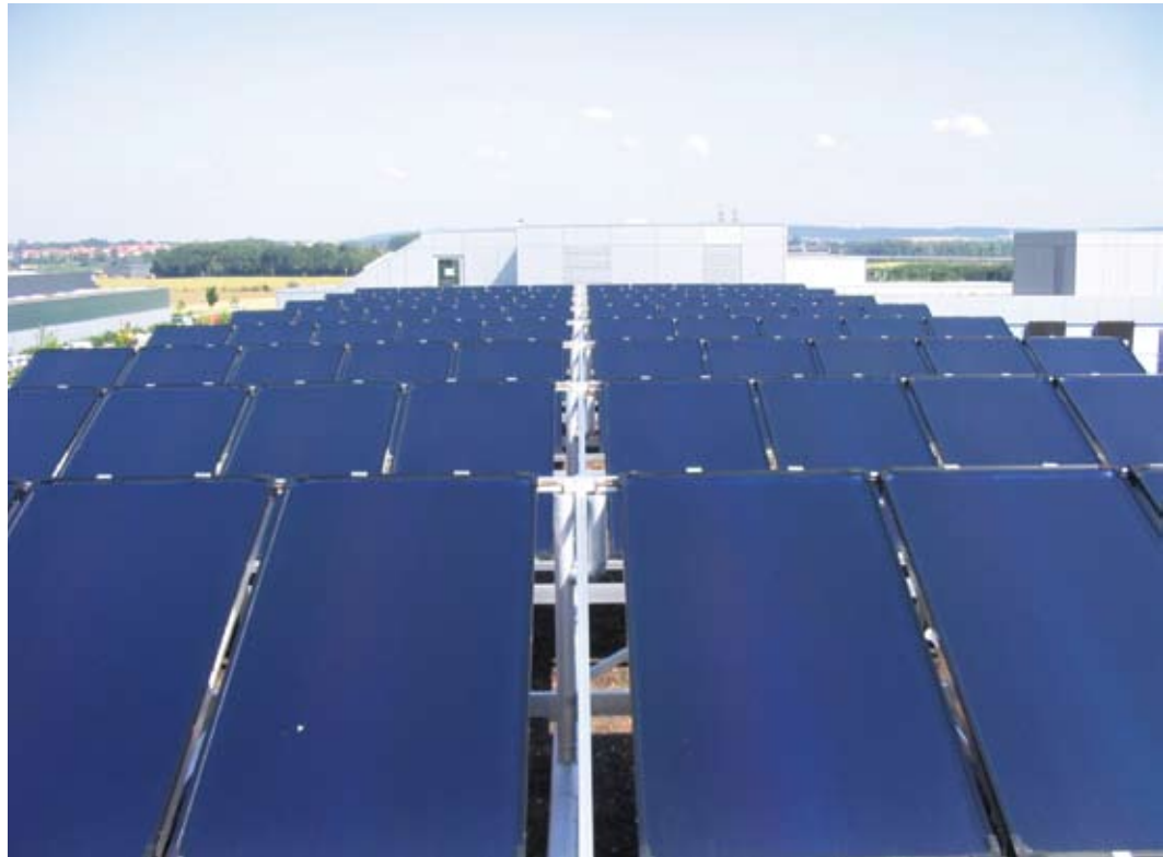
Audi installed a solar cooling system (above) at its training center in Ingolstadt, Germany. Credit: Solahart/ESTIF.
