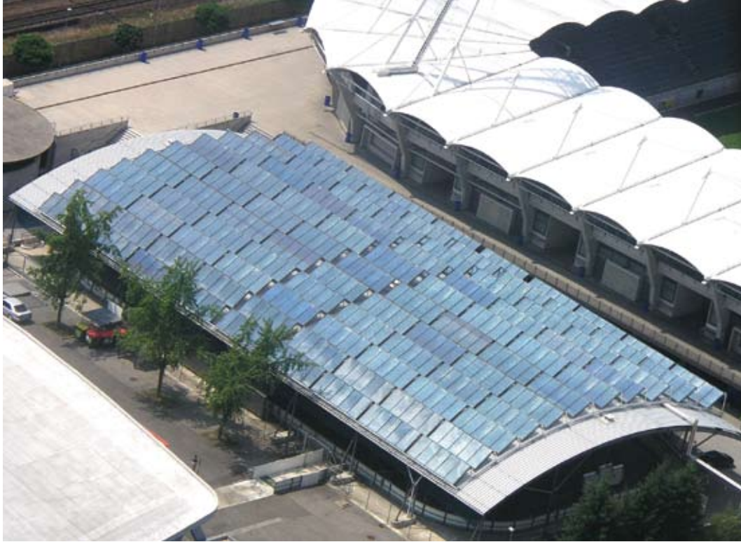
This solar thermal array, installed at Arnold Schwarzenegger Stadium in Graz, Austria, provides heat for the town's district heat system. Credit: SOLID/ESTIF
