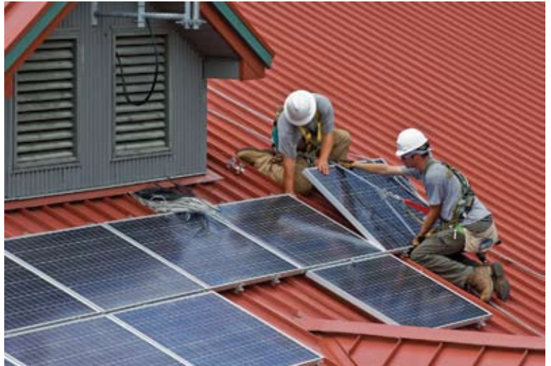
Workers install solar panels on the roof of the supervisor's office at Wayne National Forest in Ohio. Many office buildings can take advantage of solar energy. Credit: Alex Snyder, Wayne National Forest
