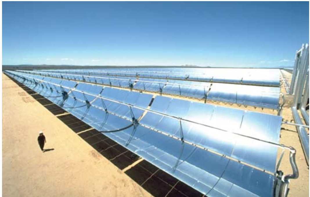
Parabolic trough concentrating solar power plants, such as this one in California, have the potential to generate large amounts of power in sunny areas of the Southwest and elsewhere. Credit: Gregory Kolb, Sandia National Laboratory
